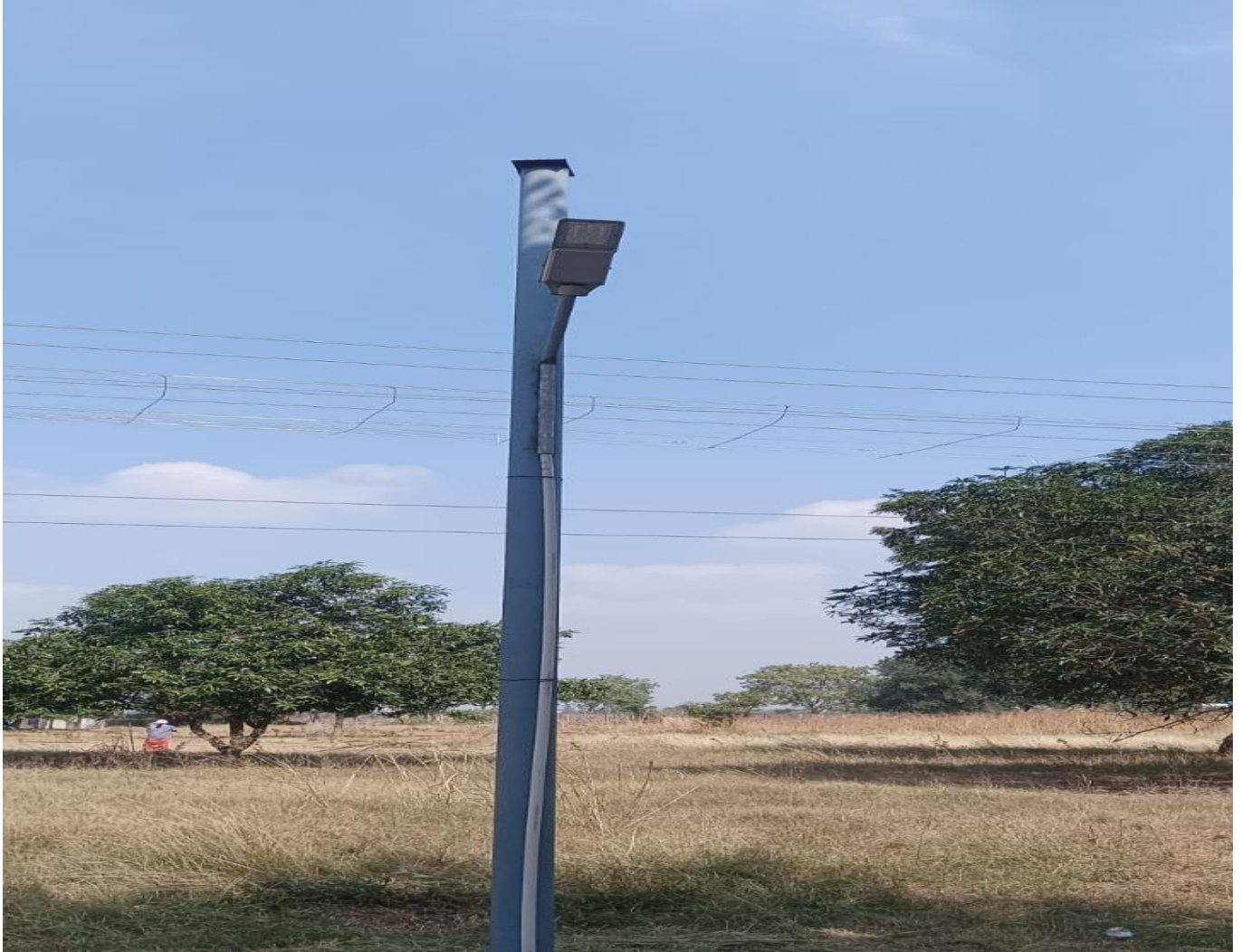
LED STREET LIGHTS
