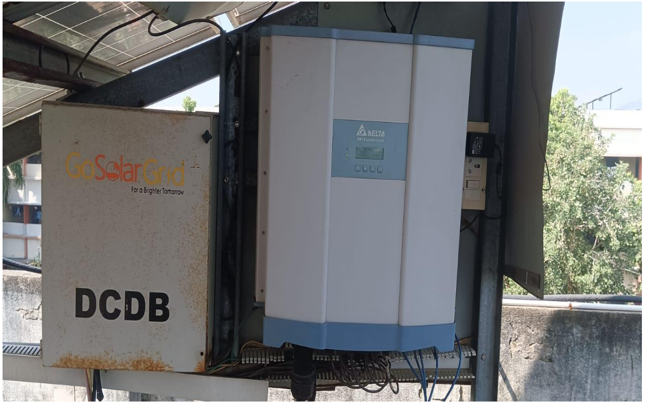
SOLAR GRID INVERTER (70 kW)
