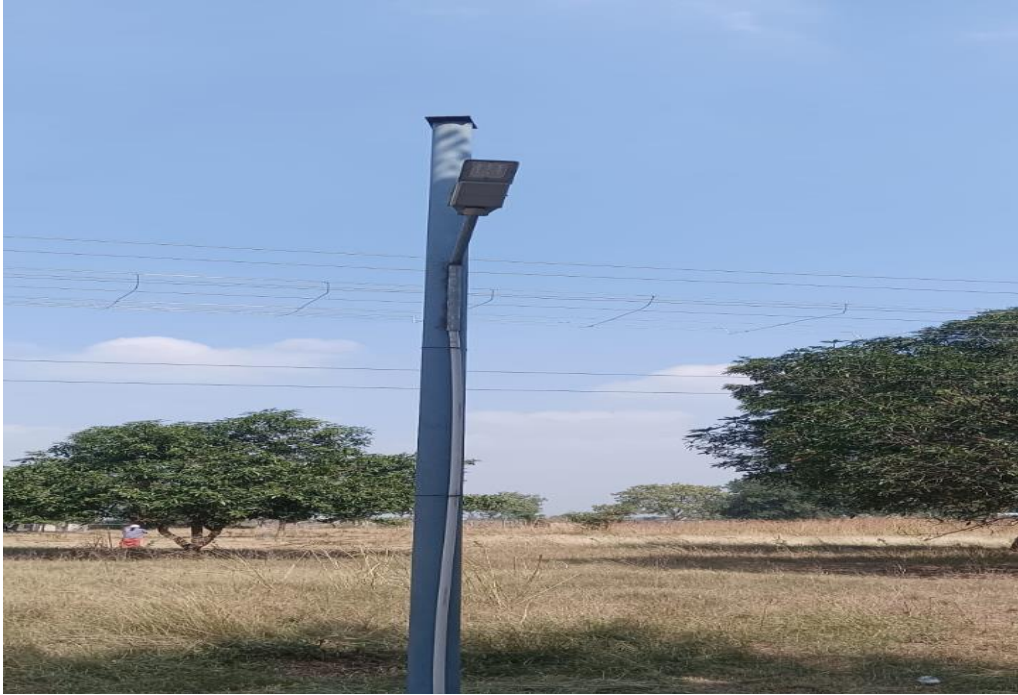
LED STREET LIGHTS
